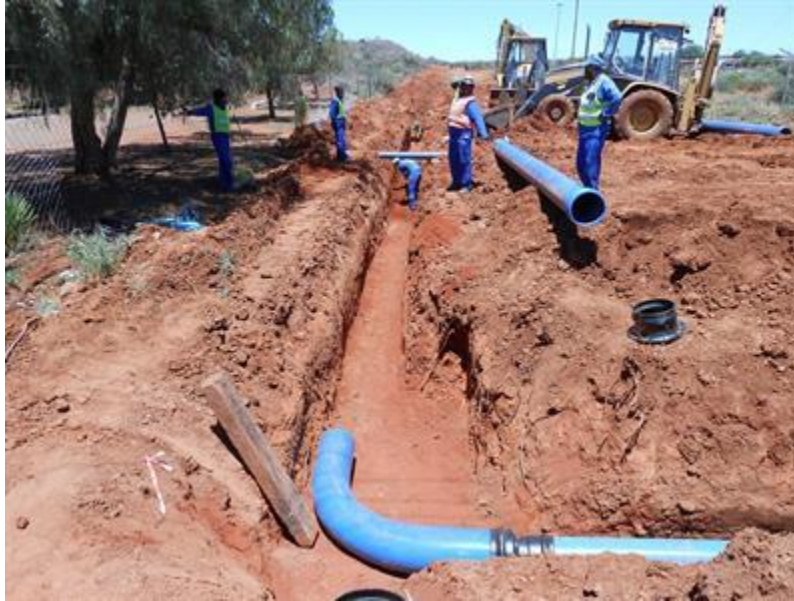
Men at work- Laying PVC Water pipes into the ground after trenching
