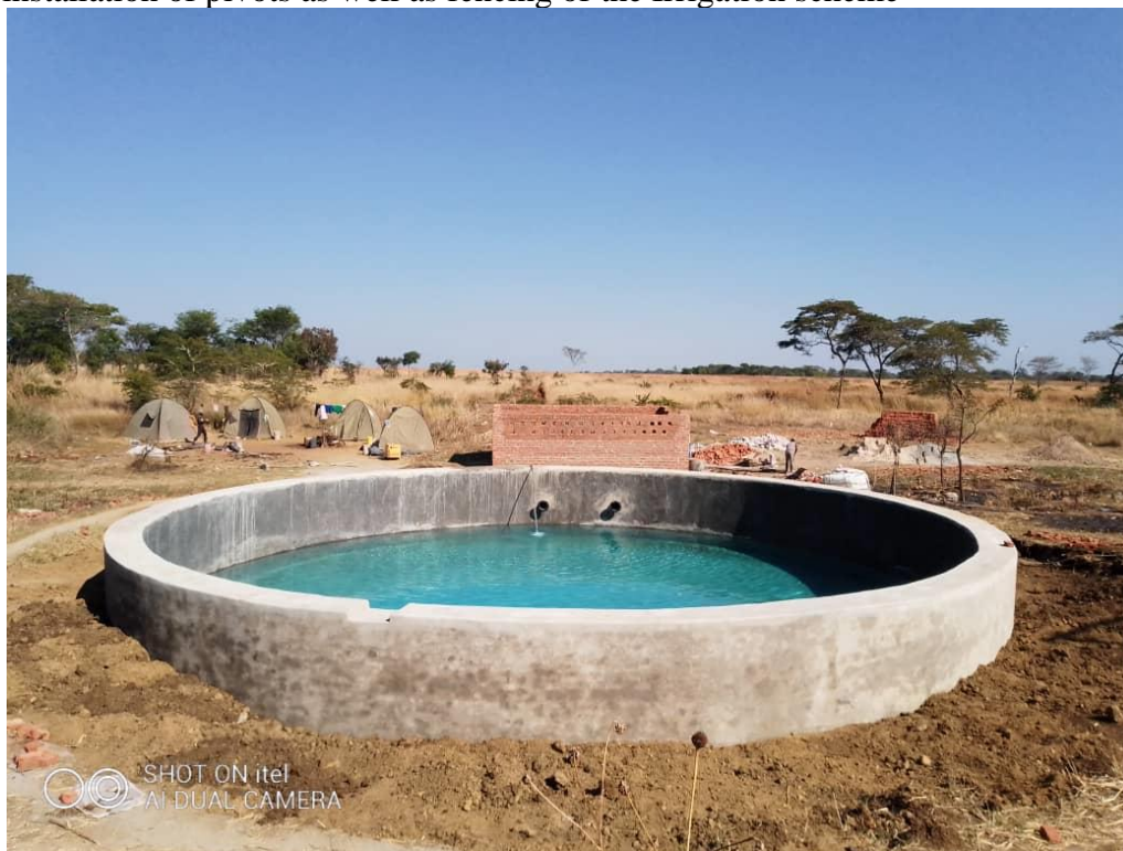
Nyabango Irrigation Scheme 500m 3 Night Storage Water Tank and pump house- Mashonaland West Province
