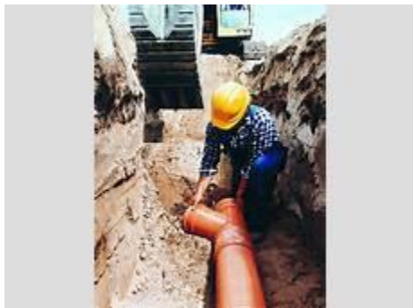
Deep in the trench and down to business-fitting a Y-Junction on a PVC pipe on a Sewer line.
